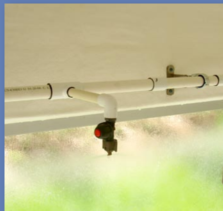
Manifold System with hardware
